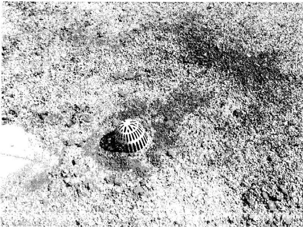
Photo 6. Deteriorated membrane in vicinity of roof drain.
